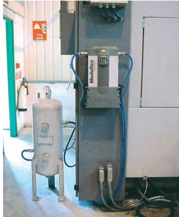
Moduflex Dry Air System installed to supply control air for a CNC machining centre
